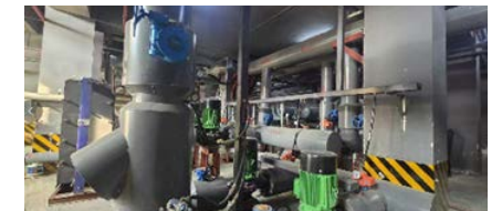
Retrofit of Waste Heat Recovery for Gas-Fired Boilers
